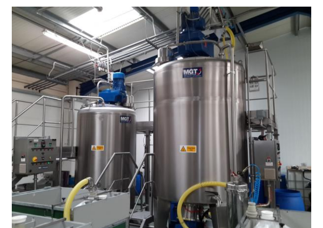
Figure 5. Mixing tanks used in the cosmetics industry. 5
